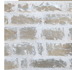
Stone: Plain, Rubble - Overgrouted
